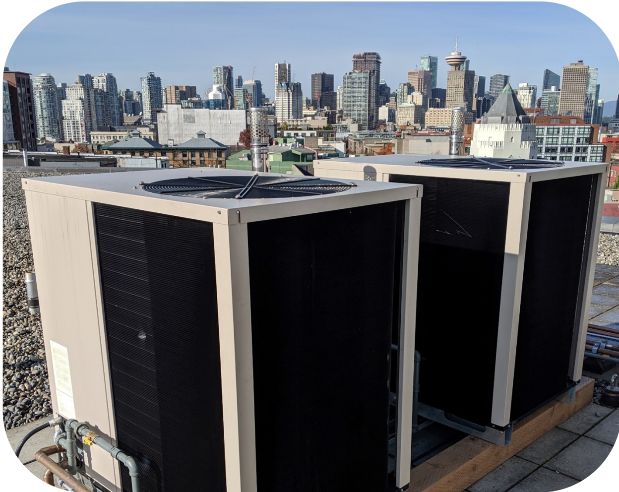
Image: GAHP units being commissioned at a facility for a FortisBC pilot project in Vancouver, British Columbia. Courtesy of Building Energy Solutions Ltd.
